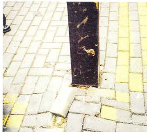
Failures in 1980s block paving of highways.
