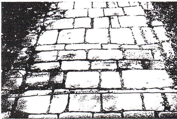
Figure 10 Hare Court, Inner Temple, detail of diagonal path. Note border stones and edge-bedded stones to save cutting and for decorative effect.
