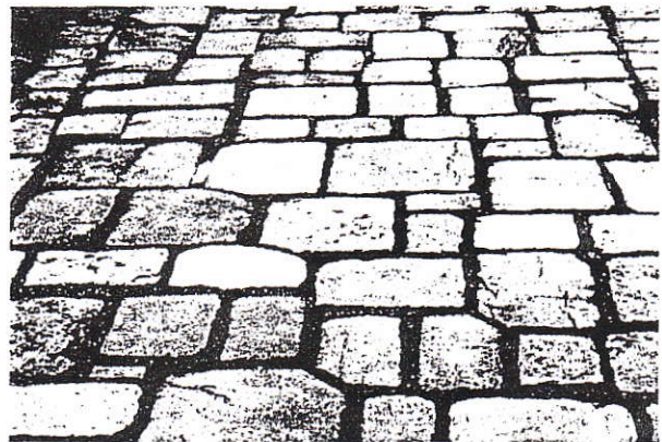
Figure 12 Staple Inn, Holborn. How not to do it: Purbeck paving laid in haphazard fashion, with wide gritty joints.
